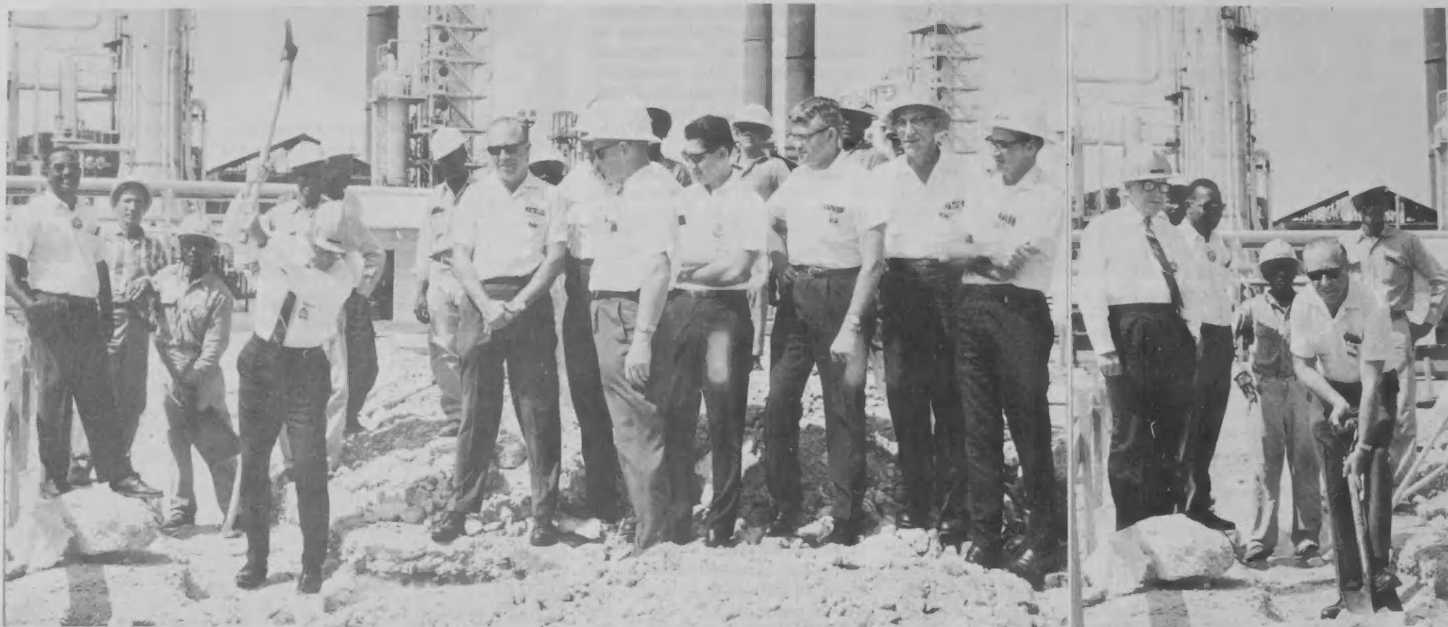
PROCESS MANAGER G. L. MacNutt (at left) performs groundbreaking work for new Control House. Attending the ceremony were the subcontractor's Project Manager E. L. Petrona (extreme left), Lago's Project Manager R. F. Morgan (8th from L), Technical Manager E. J. Higgins (11th from L), Lago engineers assigned on the project and contractor employees. At right, Mr. Morgan helps project get underway.
